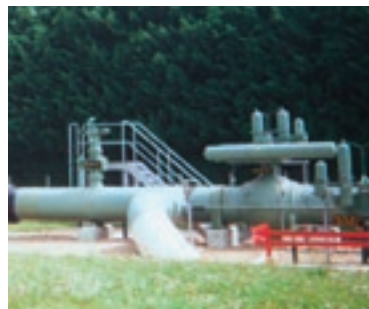
Insulating joints of pipes in gas storage
